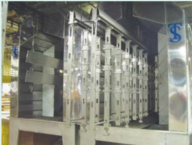
The single-stage system installed by T&S Enterprises has helped Knoll reduce CO 2 emissions by 916 tons per year while providing substantial savings in both money and man-hours.
