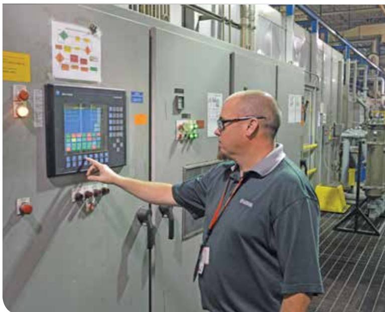
Yamaha Motor paint engineer Chet Sweatman checks the controls on the finishing line.
